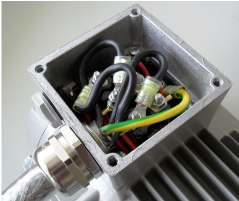
Fig. 22: Wiring on the motor connection box
