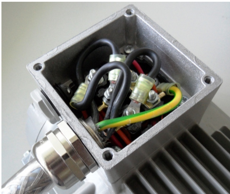
Fig. 26: Wiring on the motor connection box
